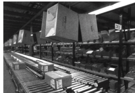
A Limit Switch in Action
