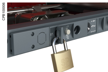
"Disconnected" position locking by padlock.
